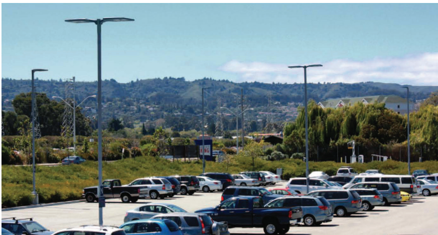
LED Parking Field Lighting Poles
